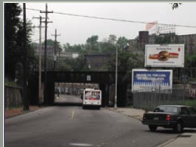
The existing and deteriorated railroad bridge over Ridge Ave. is a significant opportunity to create a positive image for the downtown shopping area beyond – requiring little more than paint, planting, and cleaning to create a memorable gateway.
